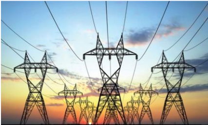
Smart Electricity and Gas Networks
